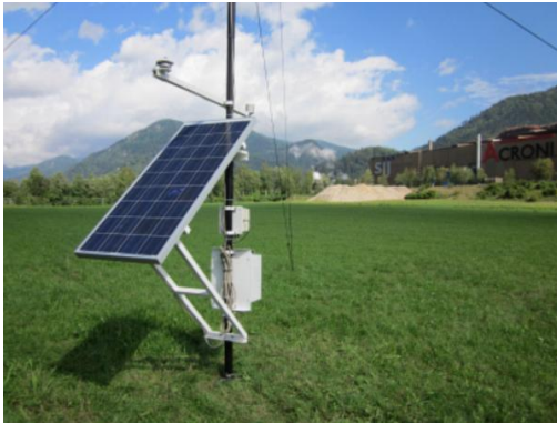
Meteorological station with a DTN router
